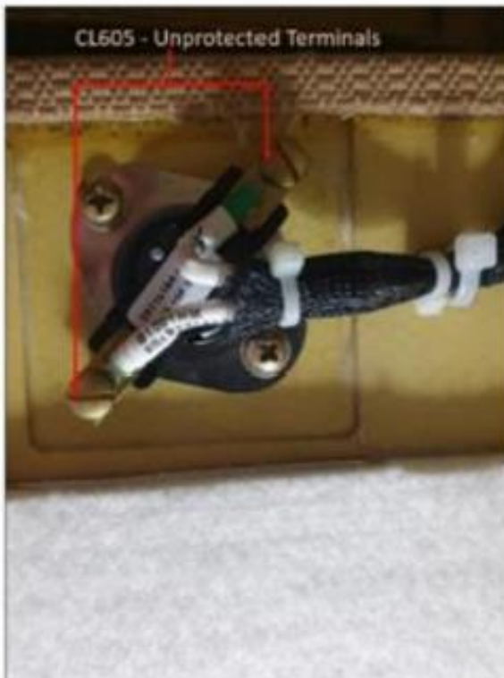
Figure 1: CL605 - Unprotected Terminals
