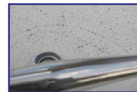
Cracks in gel coat at stanchion
