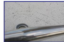
Cracks in gel coat at stanchion
