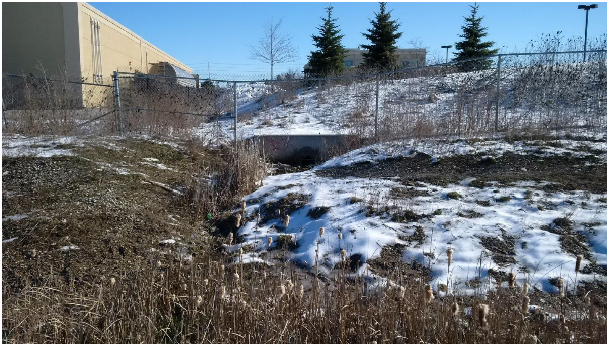
Unauthorized drainage outlet taken from the track perspective in the Greater Toronto Area
