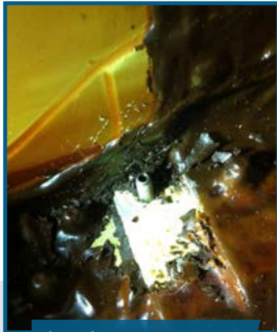
Missing Hi-Lok collar found on inspection
