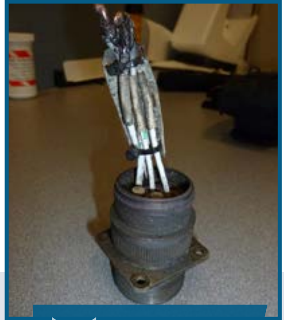
Melted propeller de-icing wiring and connector
