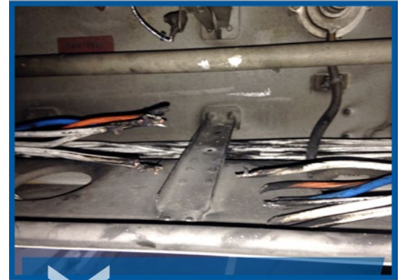
Damaged wire bundle aft of the rear spar.
