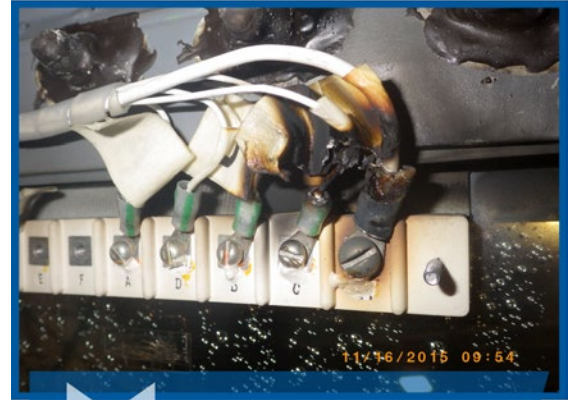
Burnt tape can be seen on the wires connected to the windshield terminal block.
