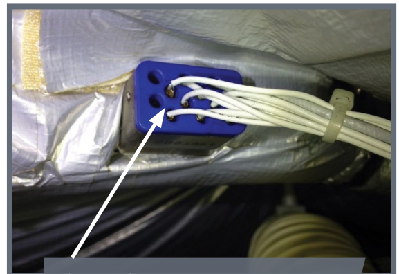
Wiring fault causing an intermittent failure of the flight data recording system
