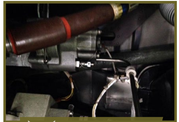
Broken P3 line at fitting on overspeed governor
