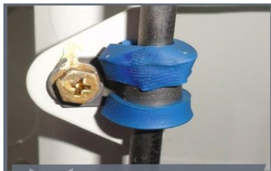
Figure 2 - Deteriorated Cushions example.
