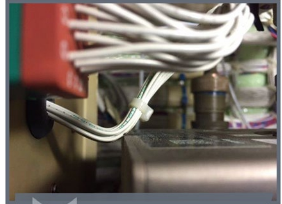
Wires touching the relay box.
