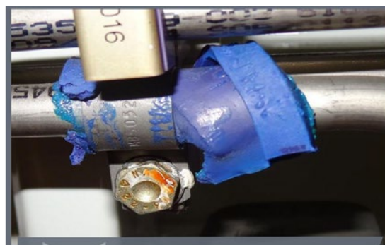
Figure 3 - Typical Deteriorated Cushion Clamps.
