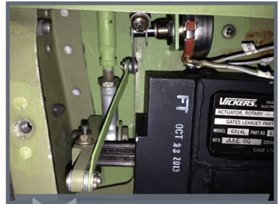
Figure 1 - incorrect linkage installation.
