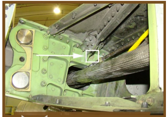
Crack found in this area, the crack was well hidden and was only confirmed with non-destructive testing
